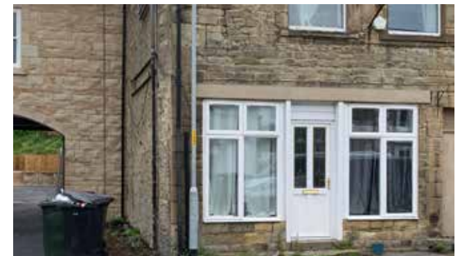
Figure 85: Good example of a former shop frontage that has been retained within a residential conversions, Shaftoe Street
