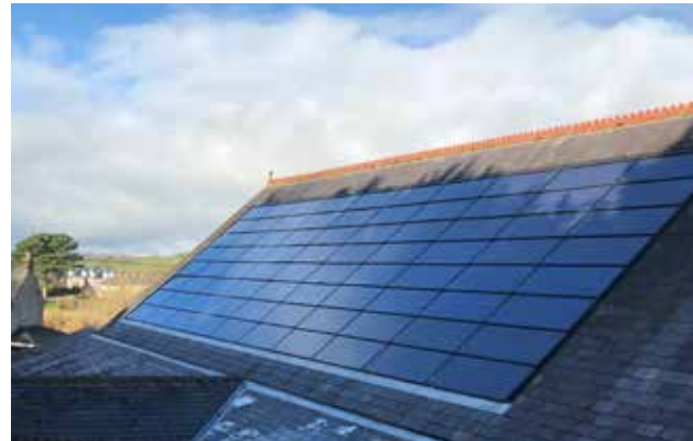
Figure 103: Solar panels retrofitted at Haydon Bridge Social Club
